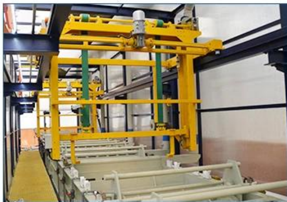
Zinc barrel plating line
