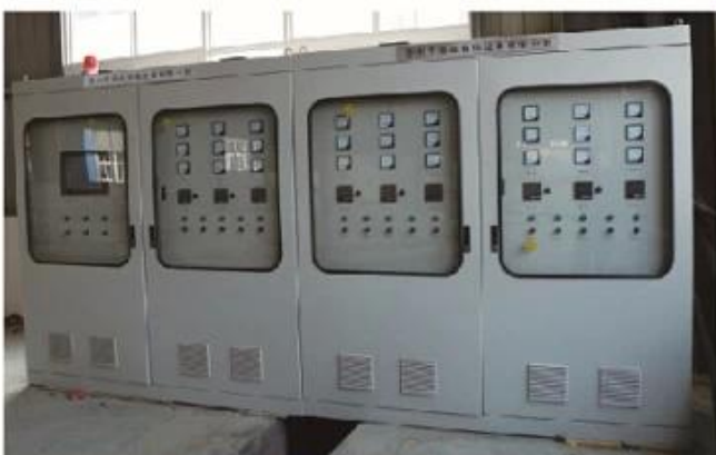
Electric Control Cabinet
