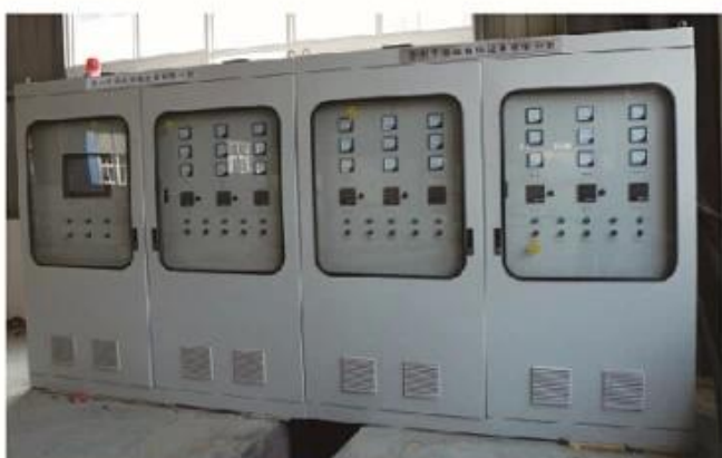
Electric Control Cabinet
