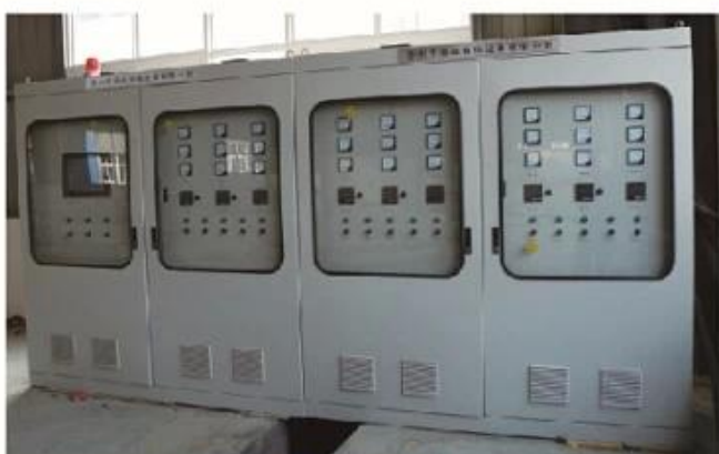
Electric Control Cabinet
