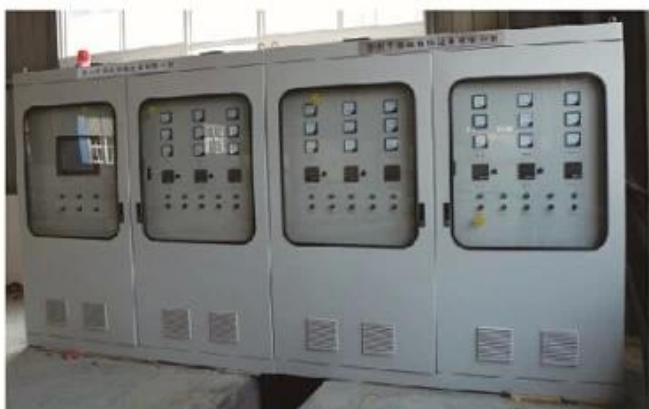
Electric Control Cabinet
