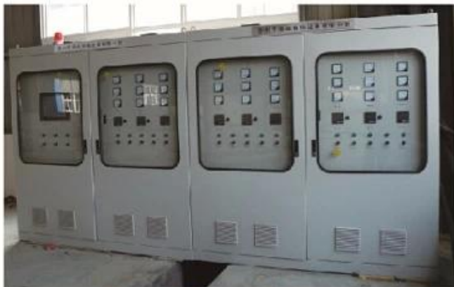
Electric Control Cabinet
