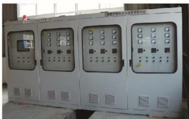
Electric Control Cabinet
