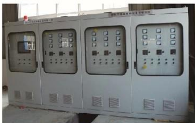
Electric Control Cabinet
