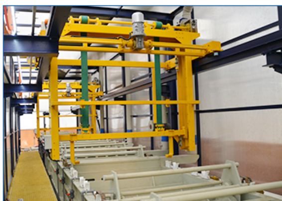
Zinc barrel plating line
