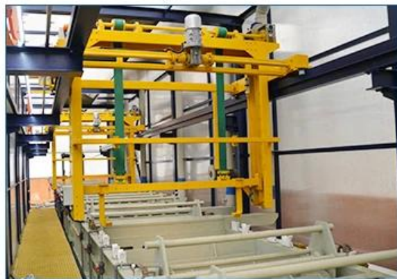
Zinc barrel plating line
