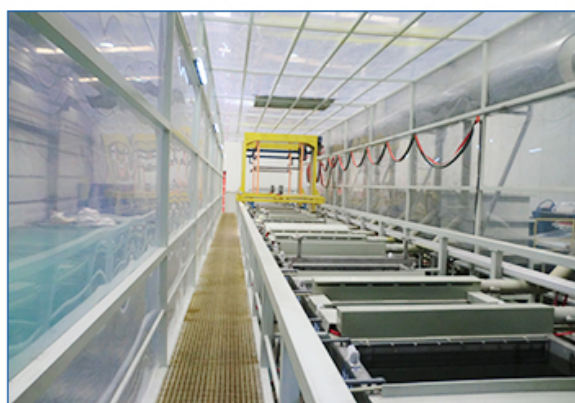
Phosphorization production line
