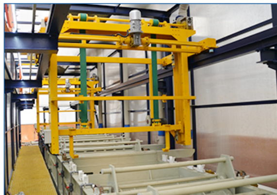
Zinc barrel plating line
