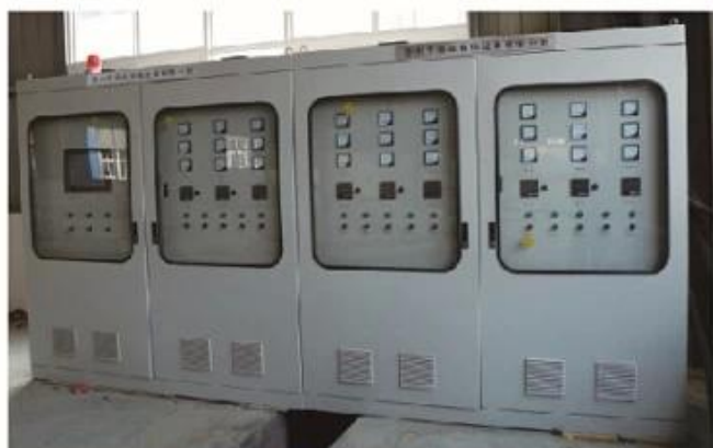
Electric Control Cabinet
