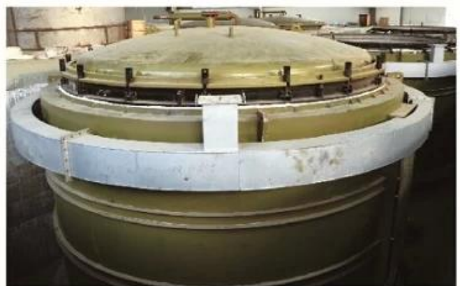
Well Type Electric Annealing Furnace (Main Furnace)
