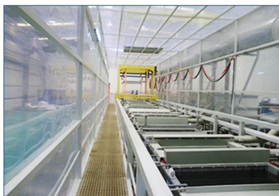
Phosphorization production line
