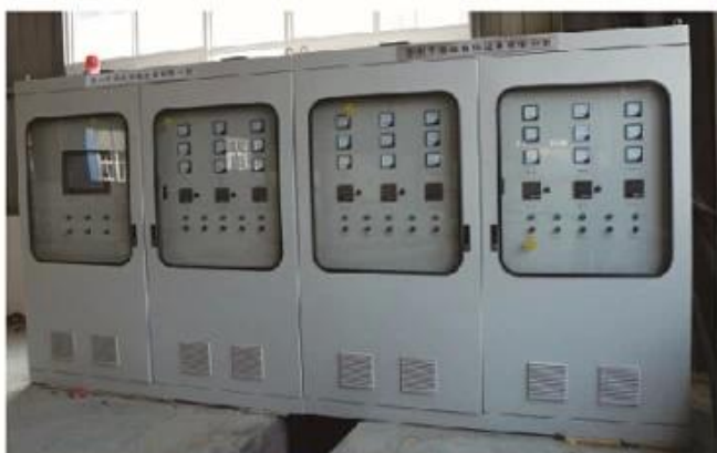
Electric Control Cabinet
