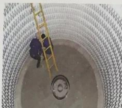
电加热炉 Electric heating furnace
