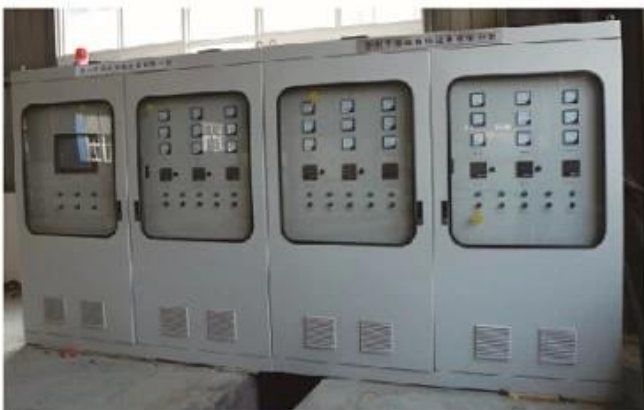
Electric Control Cabinet
