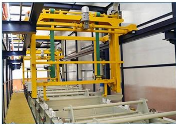
Zinc barrel plating line
