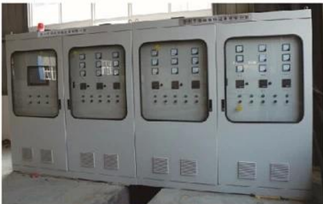
Electric Control Cabinet
