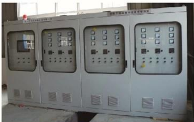
Electric Control Cabinet
