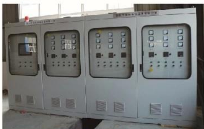
Electric Control Cabinet
